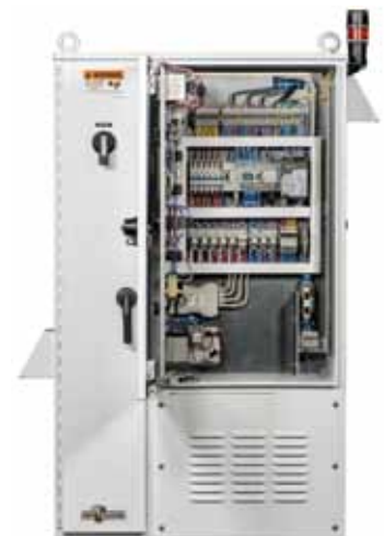
Zone 3: Controls Compartment
