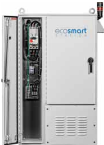
Zone 1: Service Entrance Compartment
