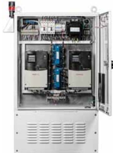
Zone 2: MCC Compartment
